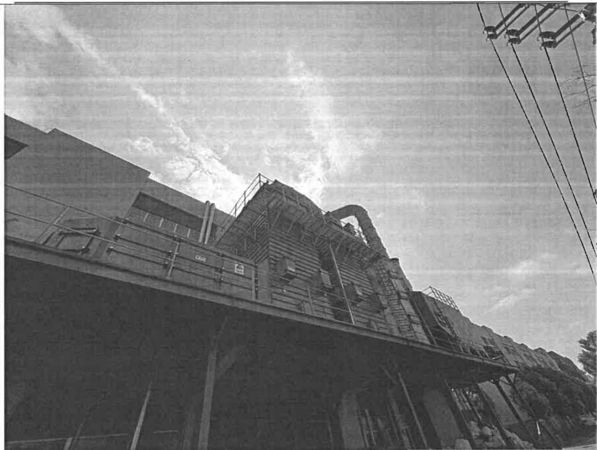
间接冷凝+二级高压静电+二级水喷淋（后端配备除雾器）+干式过滤+活性炭吸附
